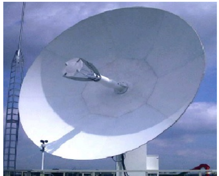
Fig. 9. X-band dish antenna at Murezeg station
